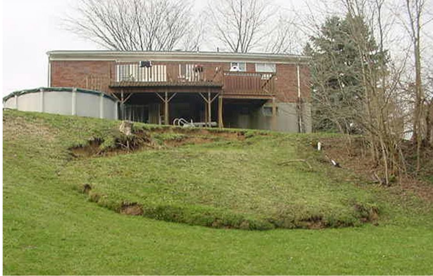
Photo of a small but typical residential landslide. Note the ground cracking at the top (scarp), and ground bulging at the bottom (toe), and the general downward and outward movement of earth.
