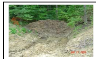
Mulch/woodchip berm acting as dam in the drainage swale to function as a temporary sediment trap.
