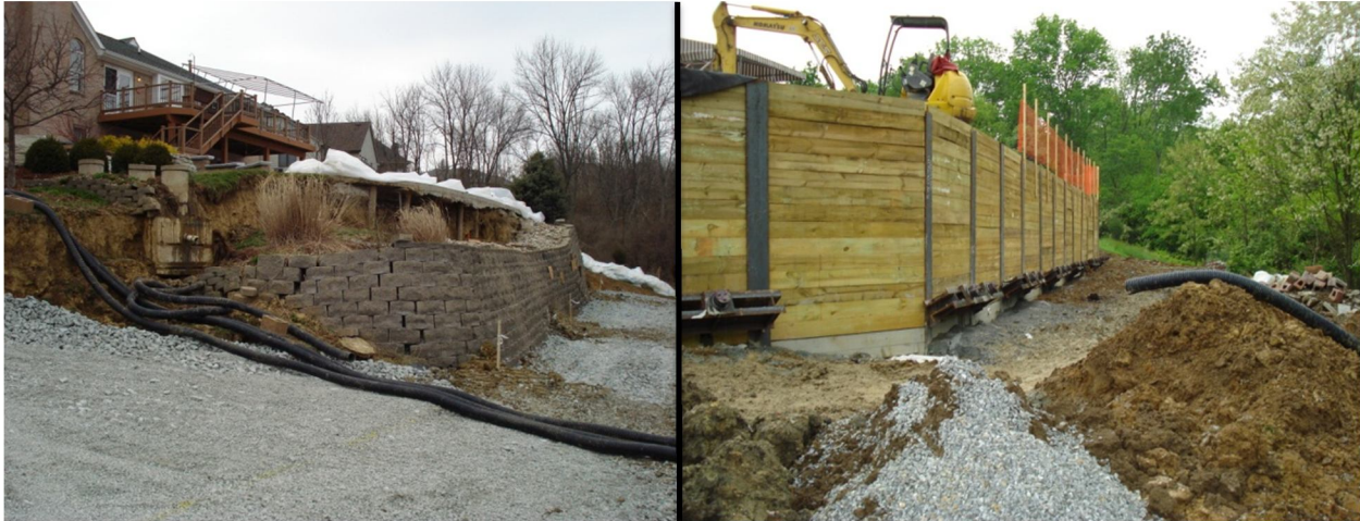
Results of a residential slope failure (left). Engineered repair of same (right).
