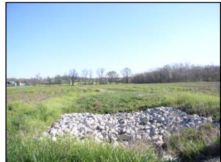
Installation of a grassed waterway to control gully erosion in a field
