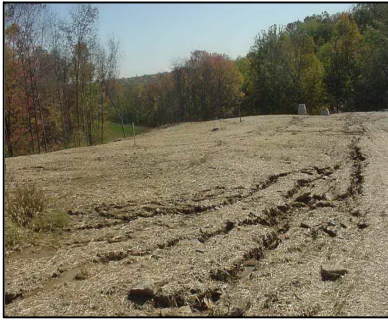
Erosion on Development site.
